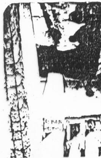
Photo 4. Spalling of concrete in column and slab
