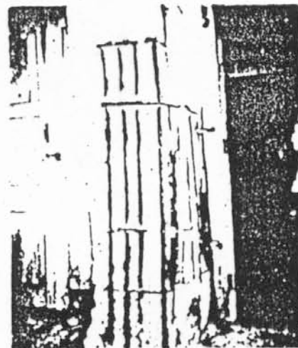
Photo 6. Spalling of concrete in column
